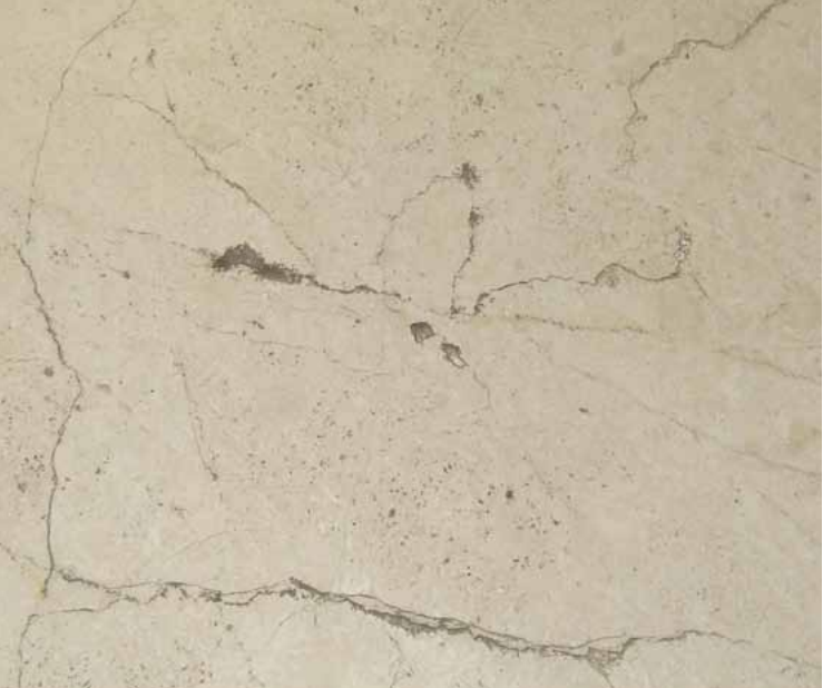
Decay of high density limestone due to unstable stylolites.
