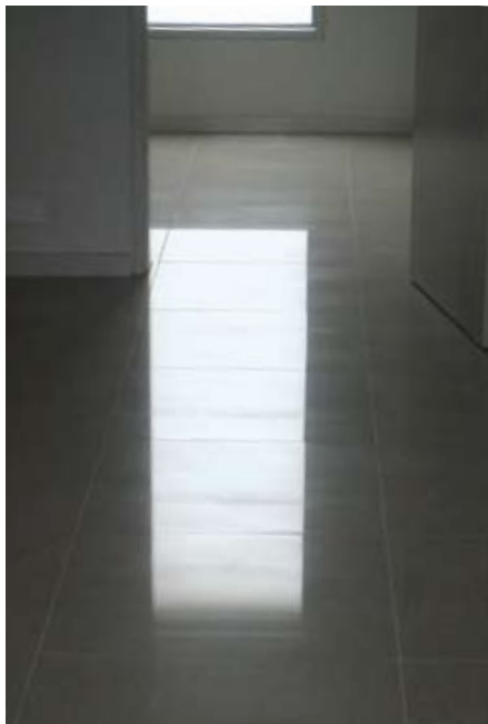
Photo No. 10. Shadowing on a floor in Sydney before treatment
