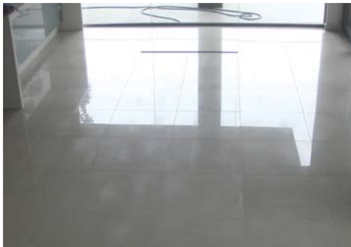
Photo No. 3 The cloudy marks on the tiles in the shaded area typifies the complaint being called "optical hazing" The tiles have a slight travertine vein running east-west the opposite direction to the hazing
