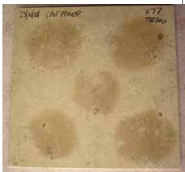
Figure 2 (right). Picture framing on marble tiles either due to adhesive or grout related moisture problems.
